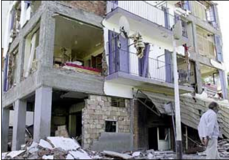
Figure 8. An RC structure affected by 2003 Earthquake in Algeria
