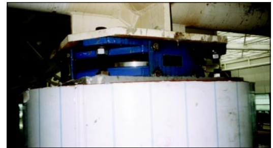
■ Friction pendulum devices were installed to seismically isolate the roof of the airport terminal.
