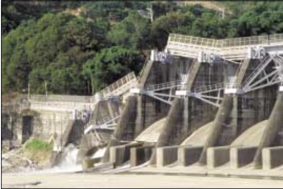
■ Figure 1. Surface faulting caused major damage to Shih-kang Dam
