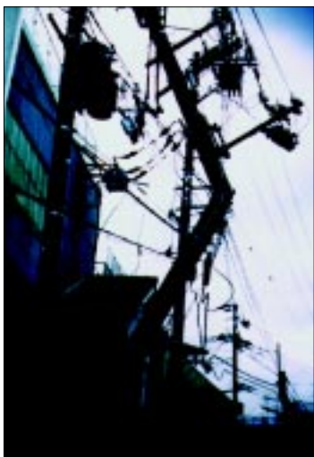
This concrete power pole was damaged following the Kobe earthquake.
