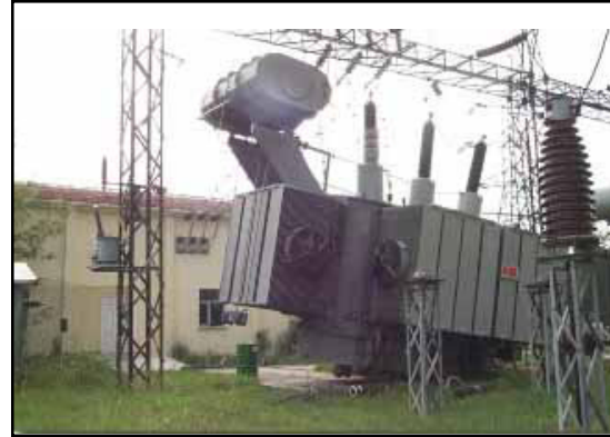
■ Figure 1. Transformer Failure During the August 17, 1999, Izmit, Turkey Earthquake (EERI, Oct. 99)
