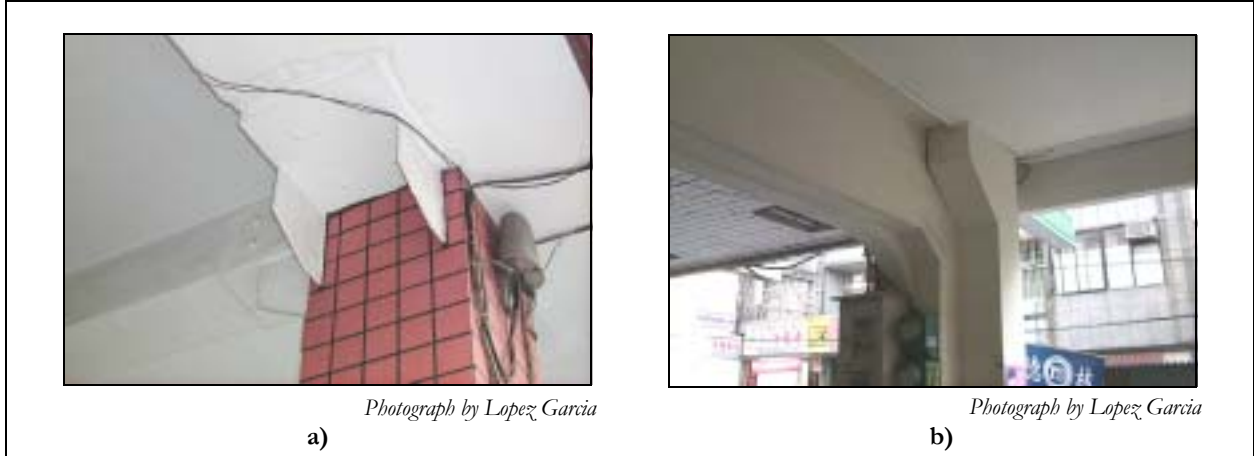
Figure 2. Non-engineered retrofit of residential buildings: (a) beam-column joint retrofitted with steel plates; (b) structure strengthened by a new column
