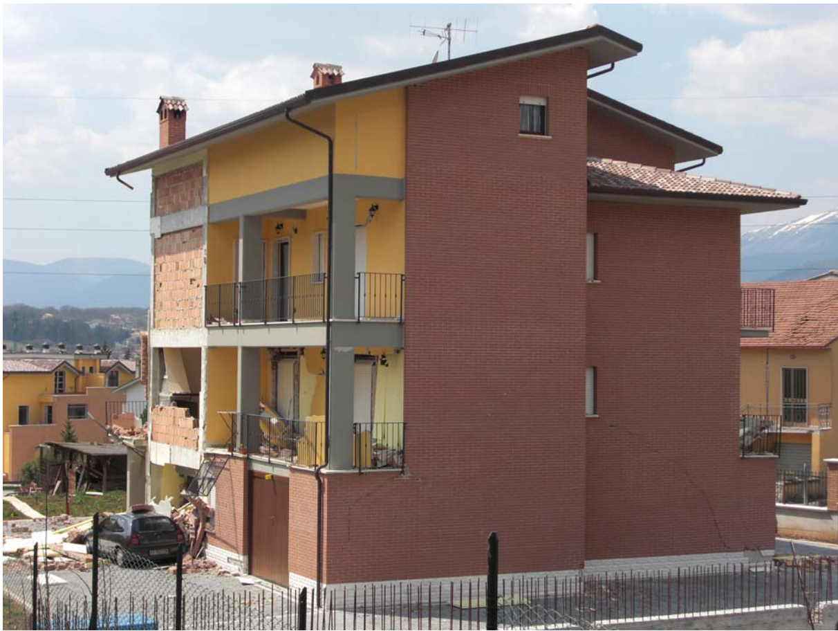
Fig. 2 Photo of the building after the earthquake. Failure of the exterior facade exposed the exterior walls made of brick. Parts of the exterior walls have collapsed crashing a car parked close to the building.
