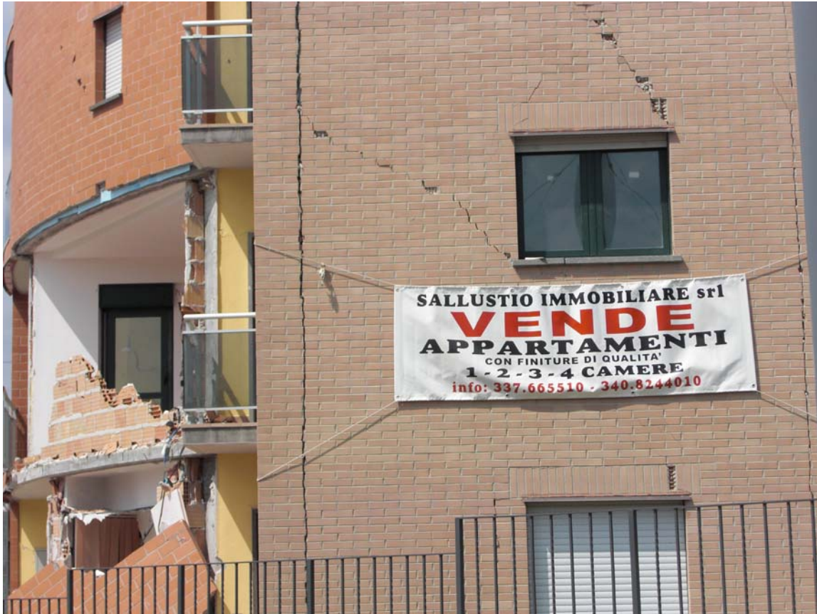
Fig. 3 Close-up view of the diagonal and vertical cracking of the exterior wall finish in the west side of the building
