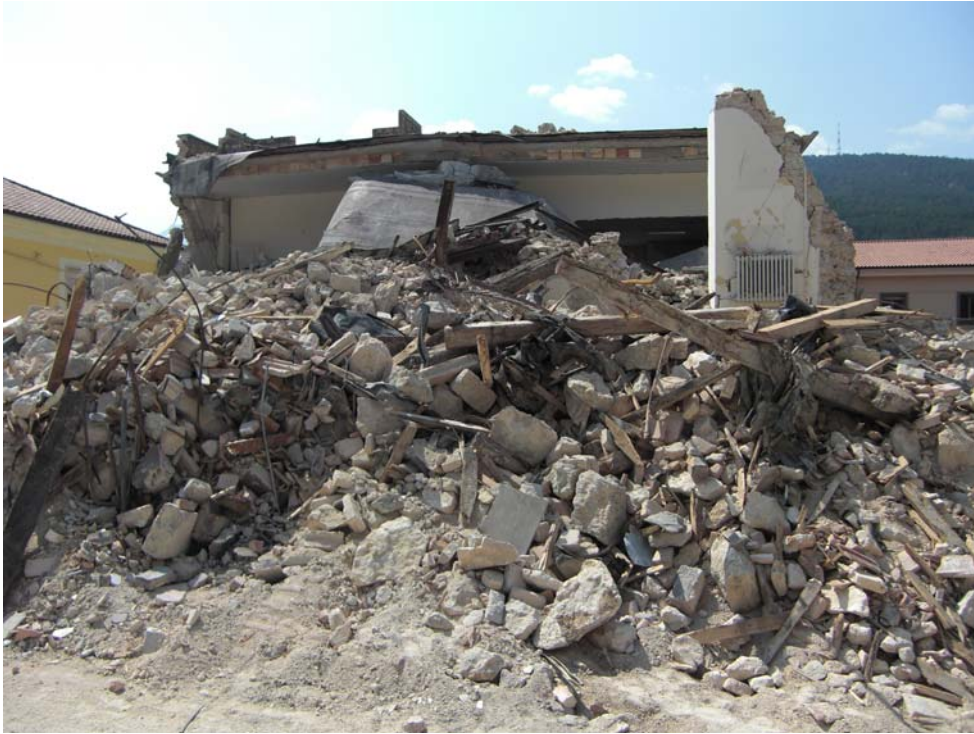
Fig. 7 Close-up view of the north side of the building. The roof slab appears to be constructed of two thin layers of concrete and bricks. No reinforcement is evident in this photo as well.
