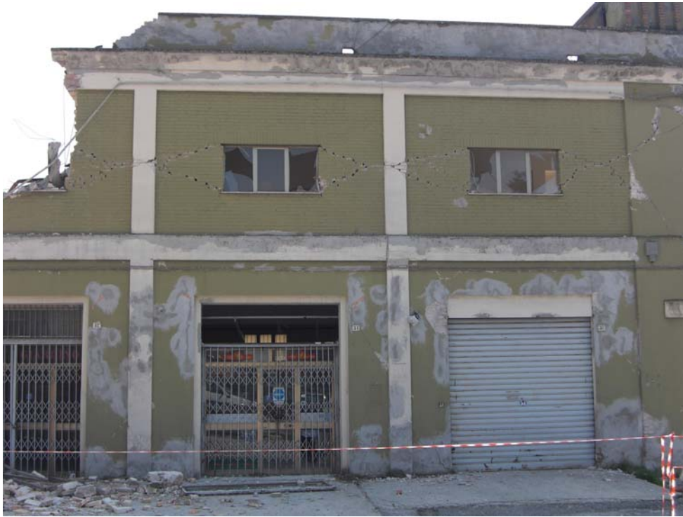
Fig. 3 Close-up view of the west side of the south part of the building. Diagonal cracking is observed across the corners of the successive windows along the mid-height of the second floor, splitting the concrete columns, as well. The first floor does not appear to suffer from significant damage.
