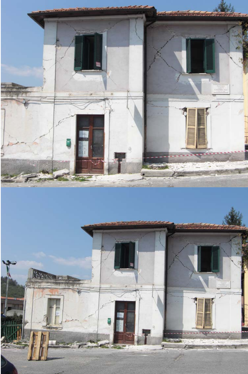
Fig. 8 Two photos of the east side of the building. Heavy damage is readily identified, classifying the structure as a collapse hazard
