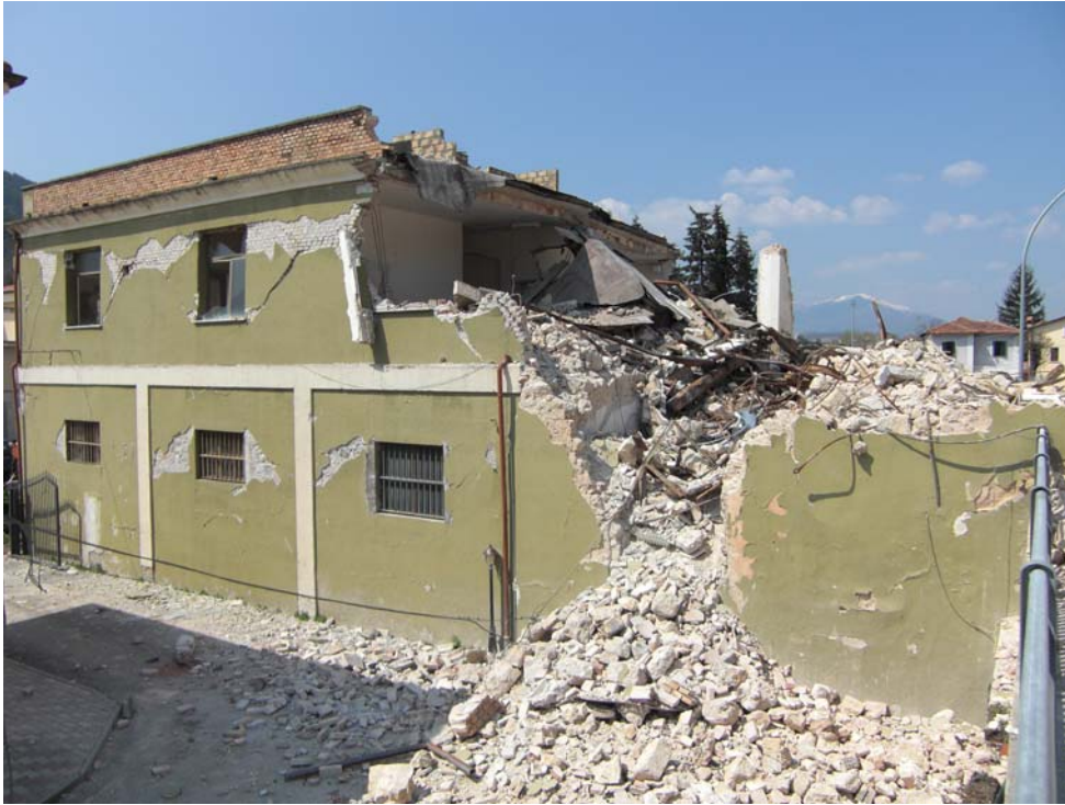
Fig. 5 View of the east side of the building. Reinforcement in concrete elements appears to be minimal; no longitudinal or transverse reinforcement bars are readily identified in the failed parts of the building
