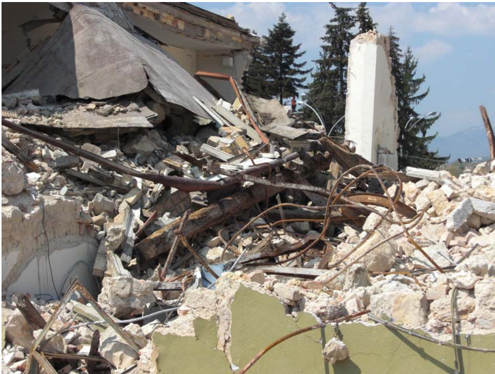
Fig. 6 Close-up view of the east side of the north part of the building, which has totally collapsed.
