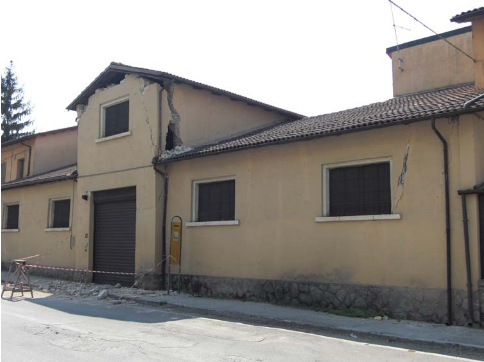
Fig. 10 General north-east (top) and north-west (bottom) views of the north side of the building. Some cracks can be identified in the adjacent one-story structures, yet no significant damage is evident in these parts of the building.
