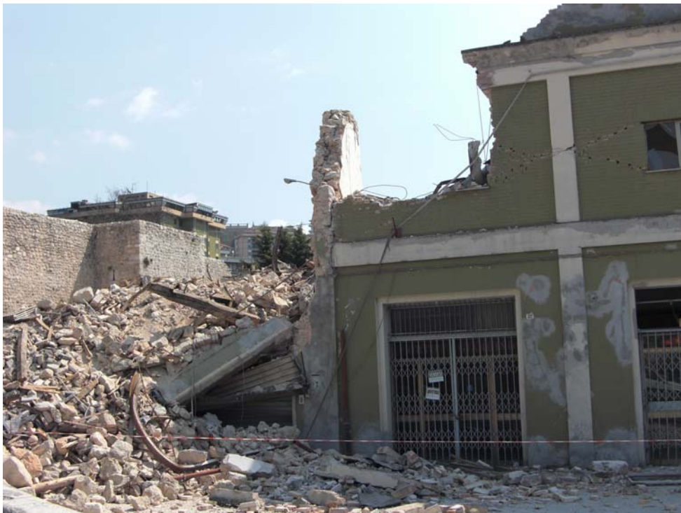
Fig. 4 Close-up view of the west side of the north part of the building, which has totally collapsed
