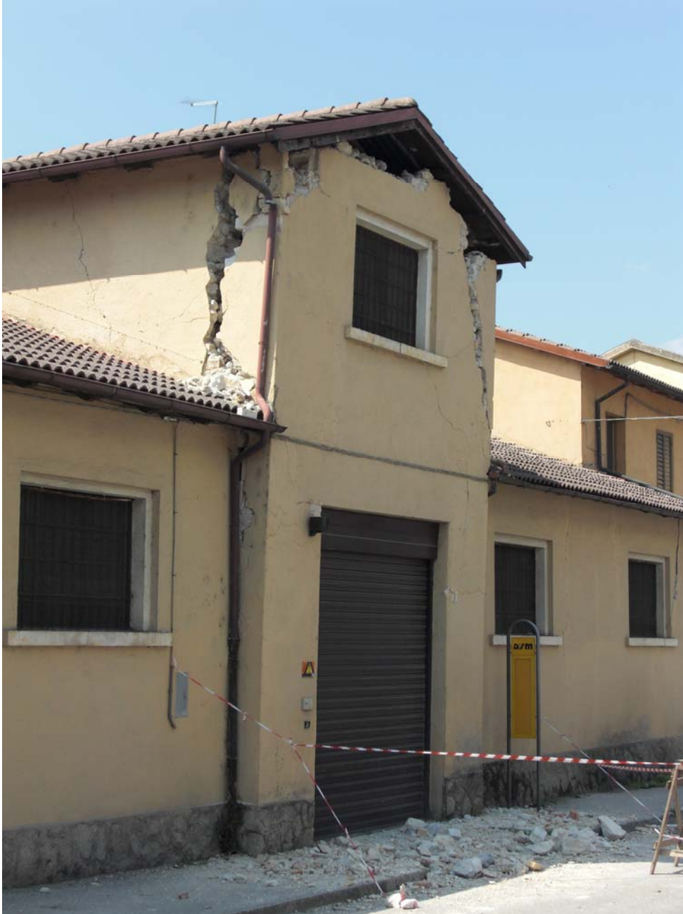
Fig. 9 North-east view of the north side of the building. Fallen debris is identified on the pavement outside the house.
