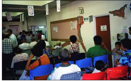
Figure 2. The first floor of the Christian Hospital remained open though the hospital suffered extensive interior damage.
