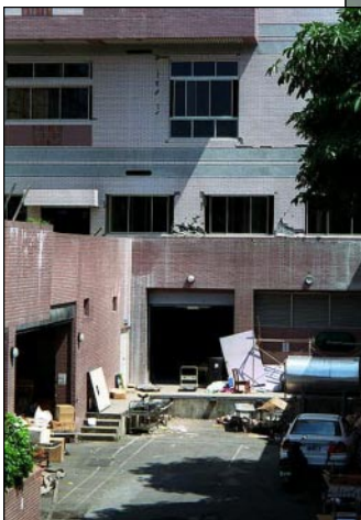
Figure 1. The Christian Hospital sustained considerable damage. Photos show (left) part of the exterior damage to the hospital; and (above) interior damage to partitions and ceilings.
