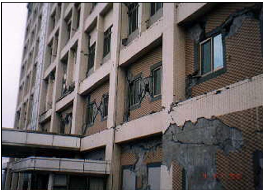
Figure 6. Damage to an exterior wall of the Shiu-Tuan Hospital in Nantou County.
